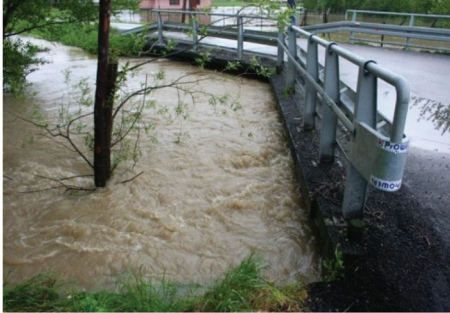
Photo 1. Flood on the Pożoga, scouring of bridges and bridgeheads – June 2010 (source: commune archives)
